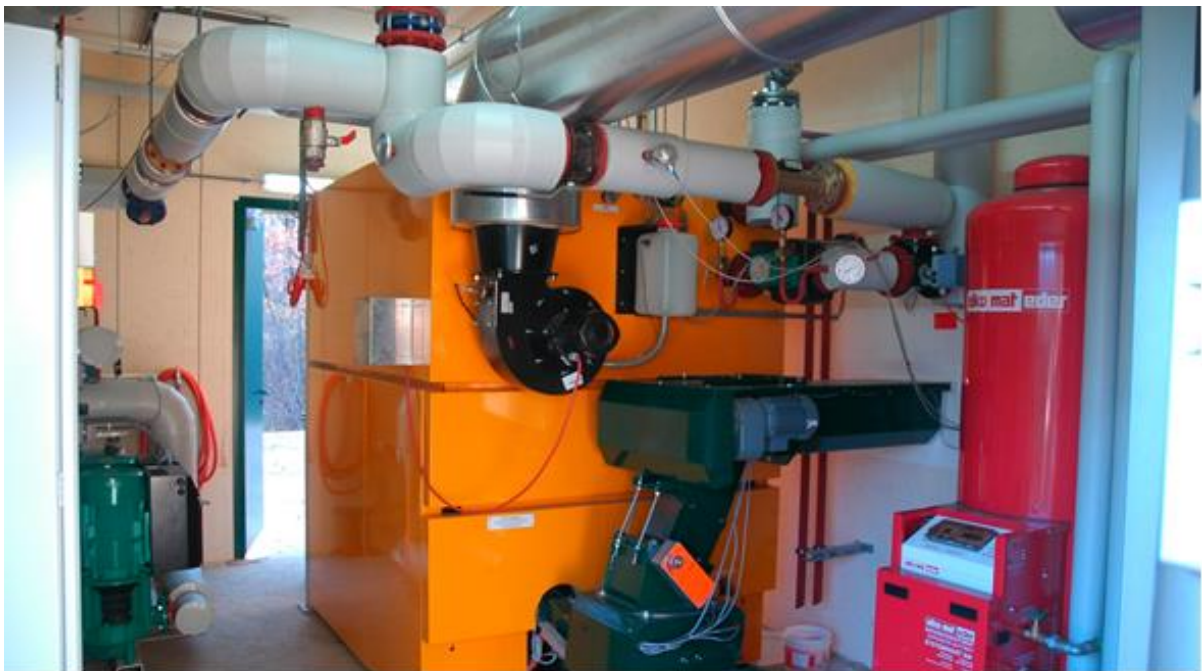
Figure 14 : Interior of a biomass micro grid heating container
